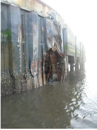
Fig.2: Damage to a quay wall after a ship collision, at the entrance to the North-Lock, Bremerhaven
